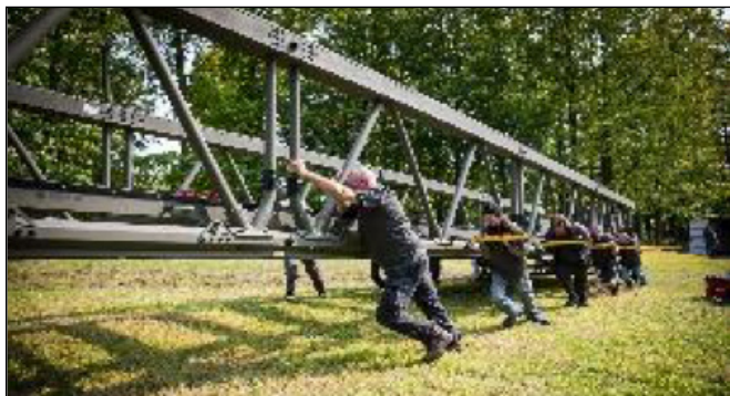
Figure 2. Only a small crew is required to set up the LVTB from one side of an obstacle.
