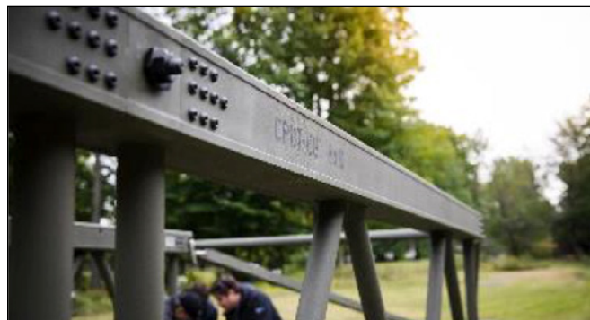
Figure 4. Sophisticated aluminum extrusions are used in the design of the top chord, enabling it to be joined without welding while still ensuring that it is structurally sound.
