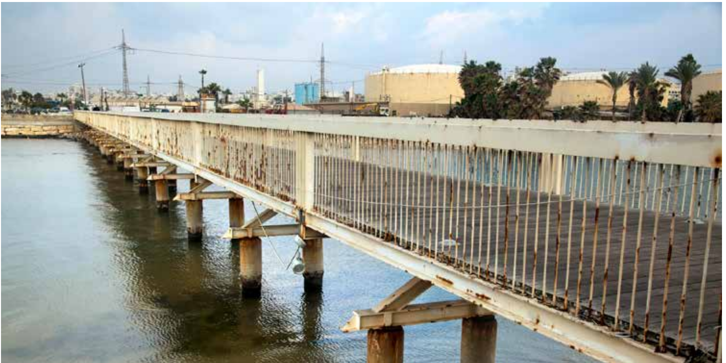
Figure 1. This rusted steel bridge beam requires costly maintenance, compared to a corrosion-free aluminum bridge.
