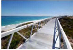
Fig 5.95 Aluminium deck of Yanchep Bridge, designed and fabricated by Peter Maier Leichtbau
