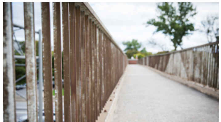
Figure 6. Corroded steel requires expensive maintenance and repairs that can be complex and harmful for the environment.
